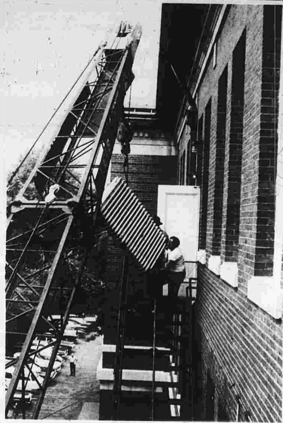
Work Starts on Bennet Heating Repairs Men of the Jack Lipman Co., of Hartford, remove an old steam radiator from the third floor of the Main Building of the Bennet Junior High School. Lipman has a $458,896 contract to improve the heating and ventilation in the four-building Bennet complex. Part of it includes replacing the Main Building's steam with hot water radiators. They hope to be done by the start of school and at least by cold weather. (Herald photo by Silver)
